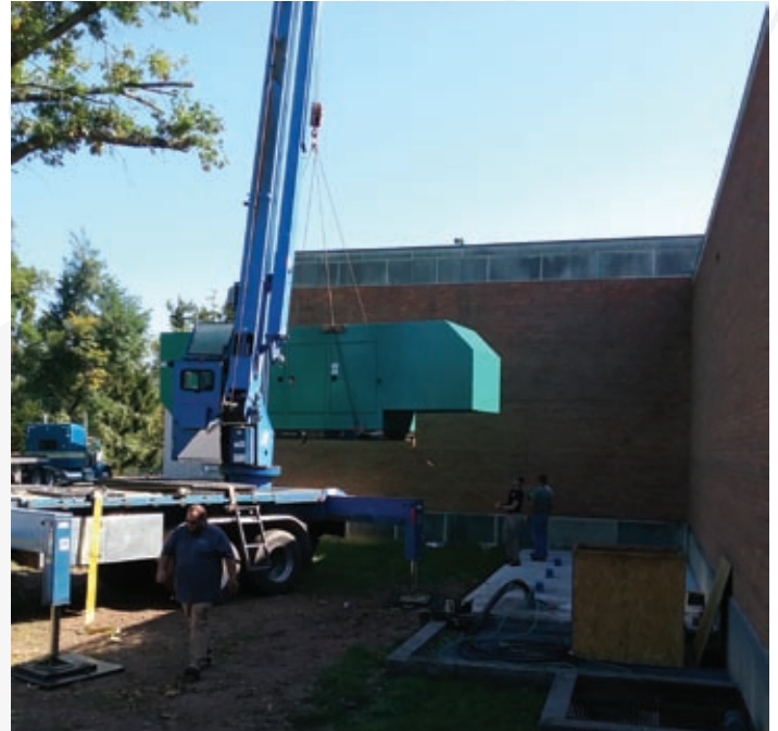
A crane is shown lowering the Huntington Museum of Art's new generator into place. The new generator provides electricity throughout the Museum during power outages. Photo by Geoffrey K. Fleming
