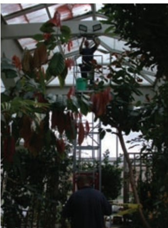
New light fixtures being installed in the conservatory. Photo by Dr. Mike Beck.
